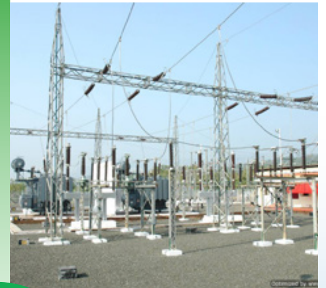
CSR inspection at South Western Railway Traction substation
