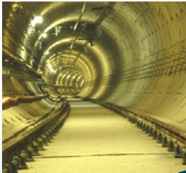
Ballastless Track inside Metro Tunnel with Zero tolerance
