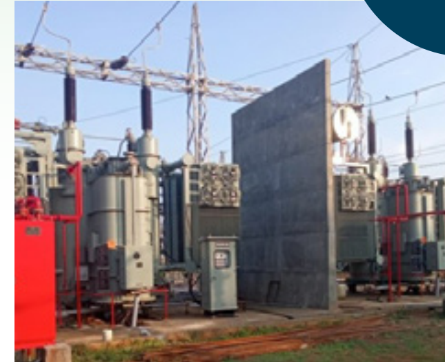
25KV Traction substation at Tambaram Chennai, Southern Railways
