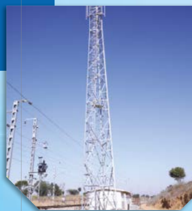
GSM-R Tower and Telecom Hut
