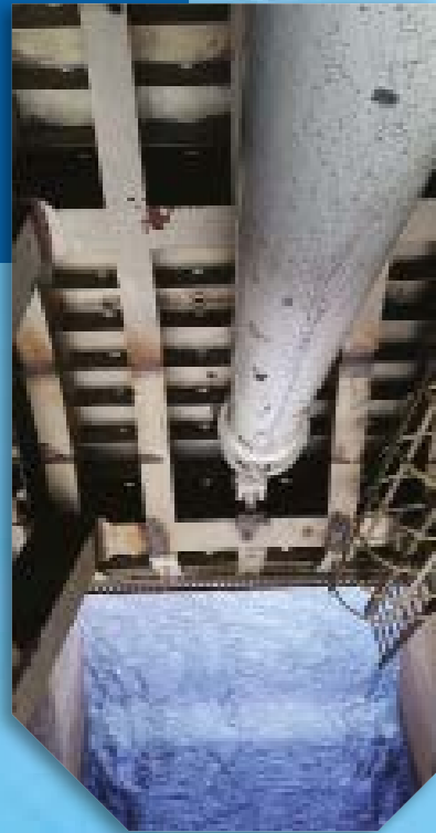
● Dam Radial Gates under operation at Tamakoshi Project, Nepal
