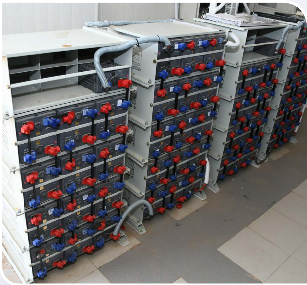
▲ Installed Power back up system in WDFC
