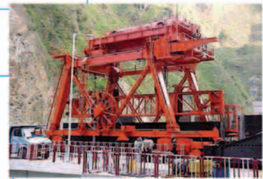
230T Spillway Gantry Crane, Chamera-II-HP
